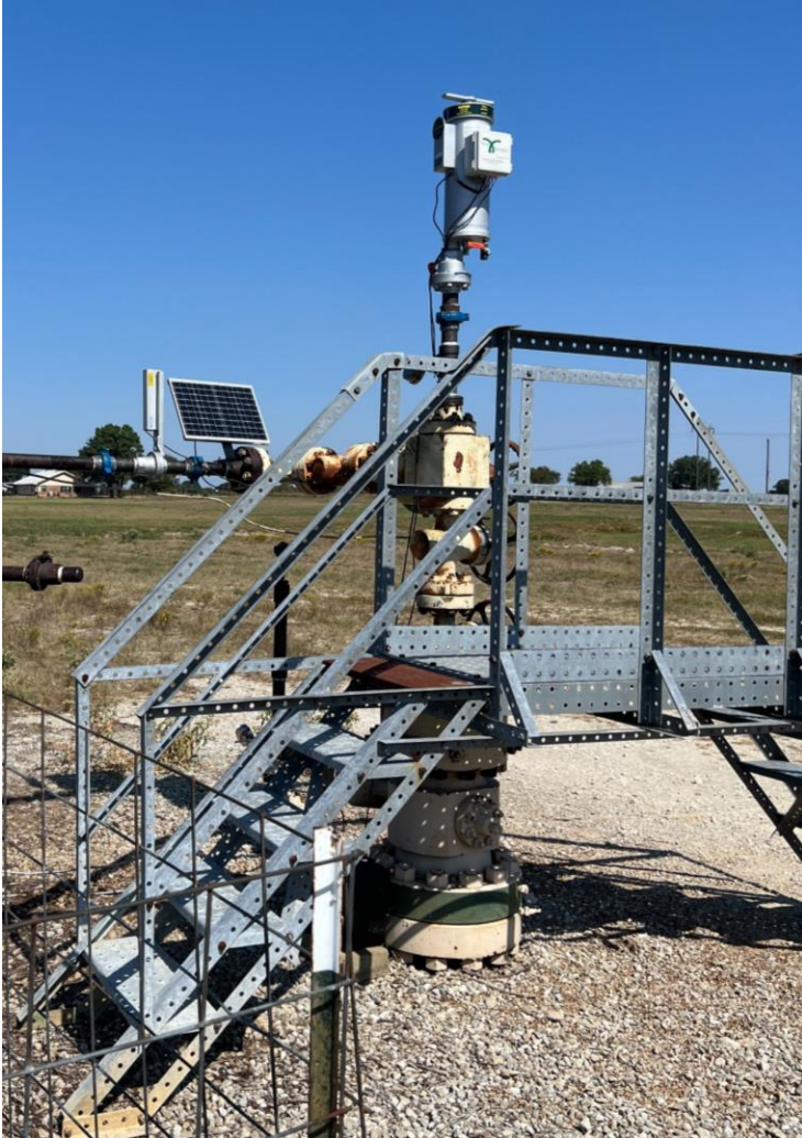
with an ABV2W for flow line control
